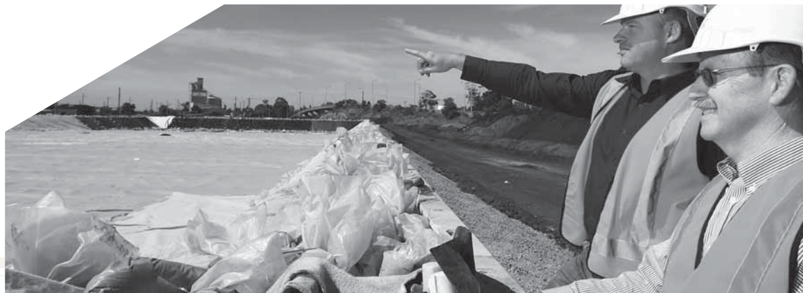
Above: Bernie Morris from EnviroPacific leads VicTrack Chief Executive, Bob McDonald on a tour of works at Spotswood.
