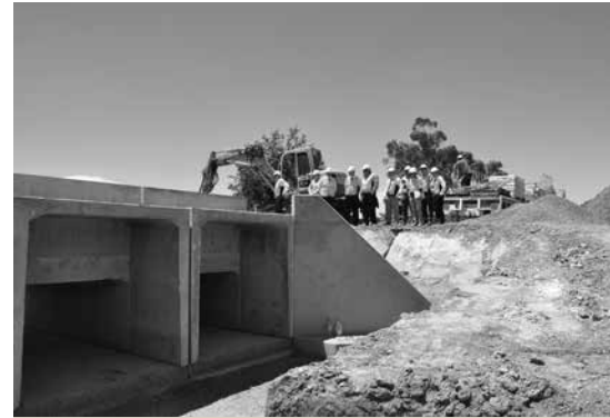
The new culverts under the rail line at Beaufort will protect the township and road and rail infrastructure from severe flooding.
